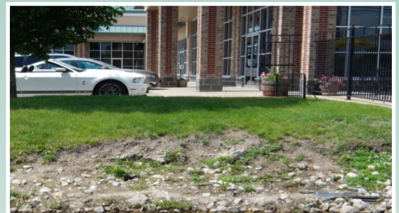
Repair exposed soils by regrading, then cover with sod or erosion control blankets or mulch and seed.
