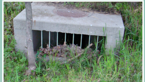
Remove debris and litter from all inlets and outlets.
